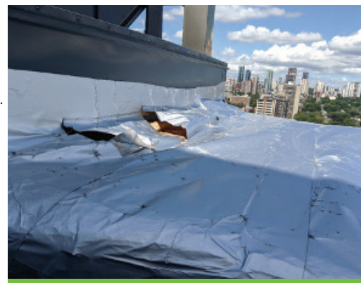
Figure 1 - Torn Insulation on a MUA Unit
